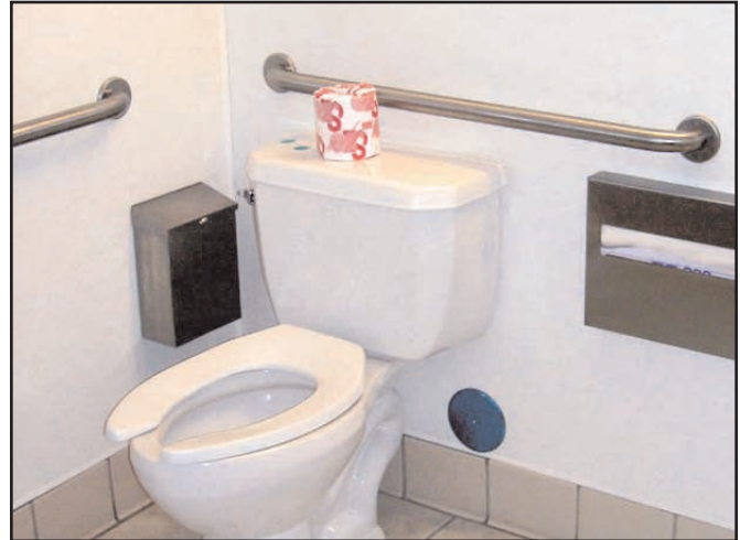
Grab bars behind and beside the toilet
